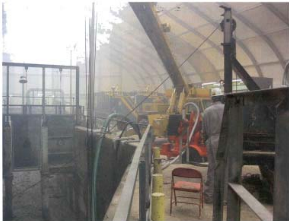
The oil-water separator as it appeared after the temporary structure was erected and most of the sludge had been removed.
