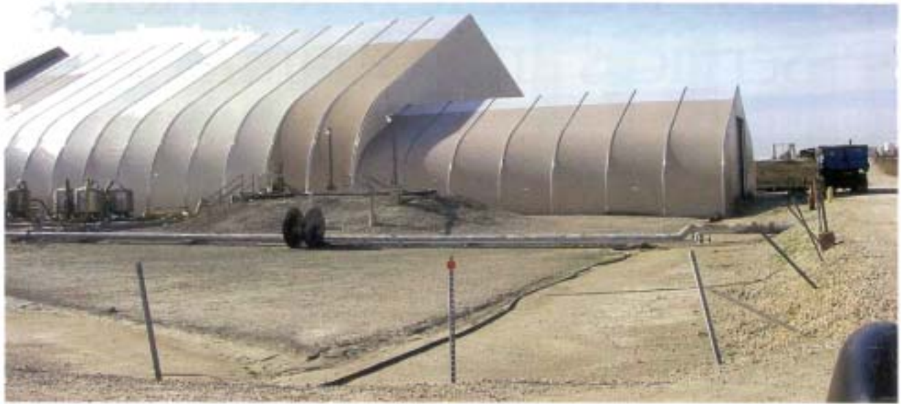
A fabric-covered temporary structure, designed to capture VOCs during the cleaning operation, completely enclosed the oil-water separator and surrounding work area.
